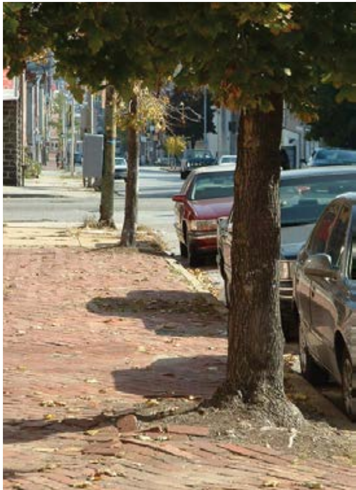
Figure 9. A common infrastructure conflict results in tree roots lifting or cracking pavement due to inadequate setbacks between trees and pavement. Photo: Edward F. Gilman
