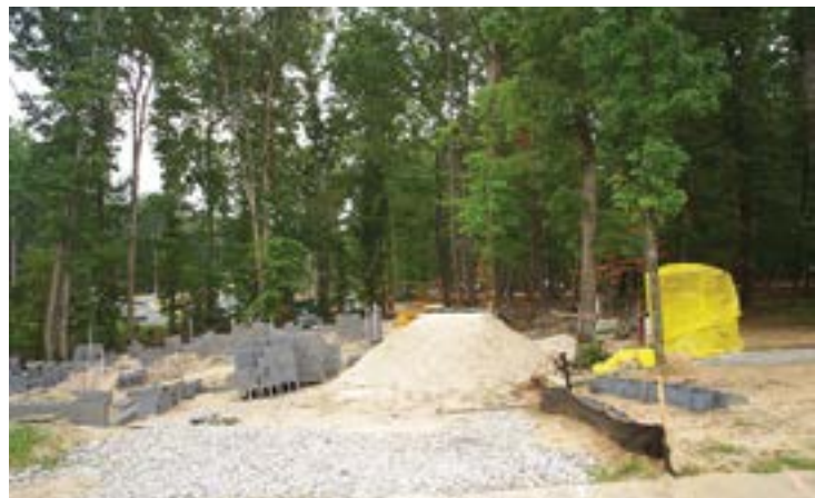
Figure 6. Improper disposal of construction materials and inadequate protection negatively impact trees at a construction site.
