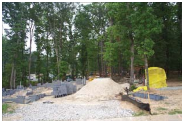
Figure 6. Native soils disturbed during construction are compacted and contain building rubble
