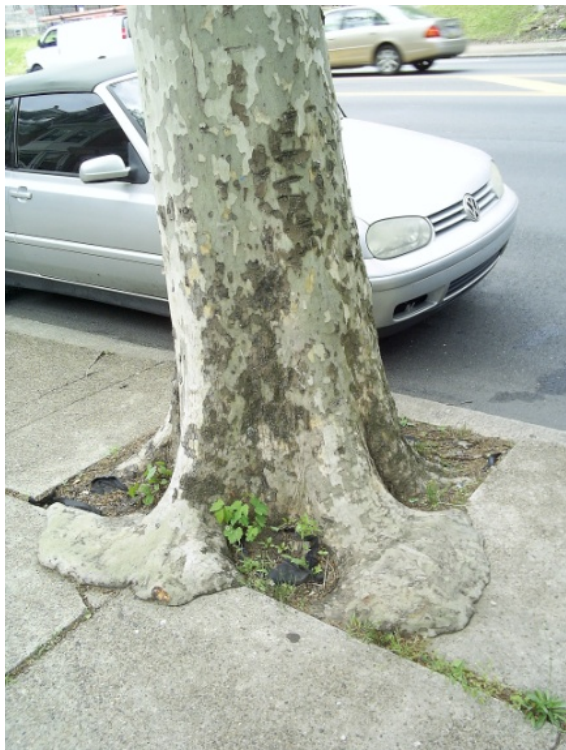
A tree that has overgrown the rooting space it was given.
